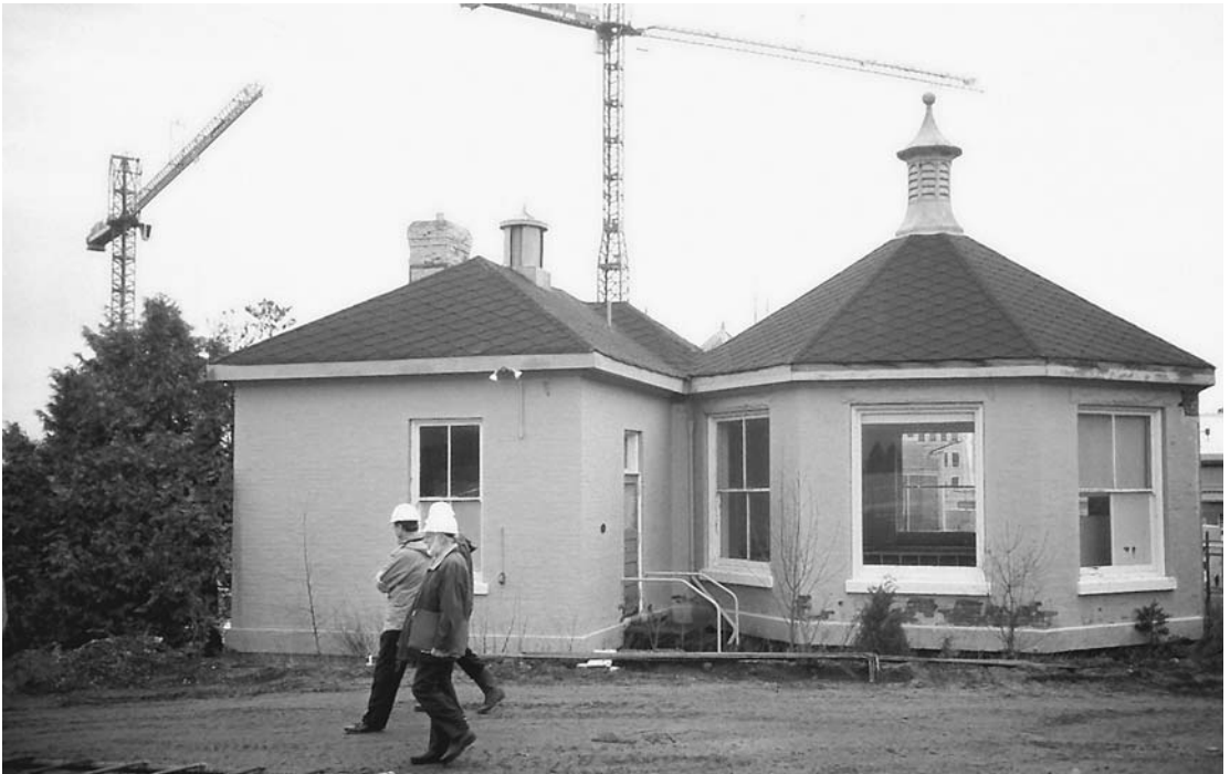
FIGURE 1.17. Pemberton operating theater.
